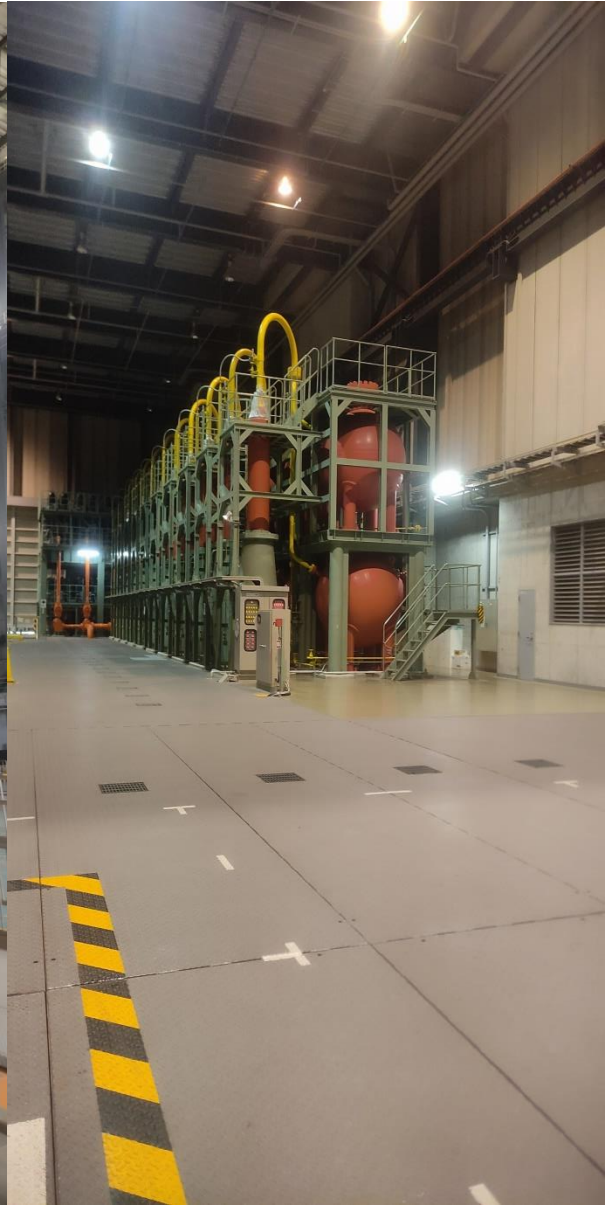
Hydraulic liquid pipes for Actuators
